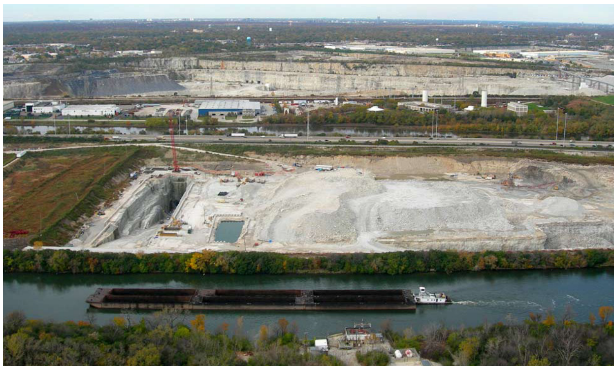
Photograph 7 : Aerial view of the Chicago Sanitary and Ship Canal, upstream of Calumet-Sag junction, near McCook Reservoir (under construction).
