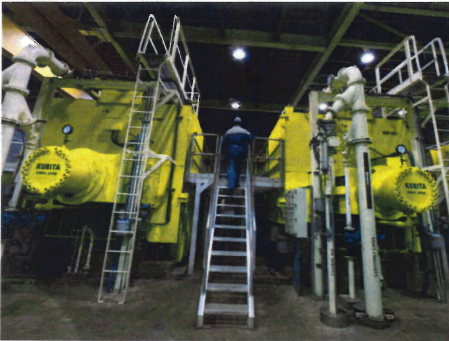
A city worker climbs onto the huge bank of racks that dry the sludge created as millions of litres of waste water are cleaned daily at the Montreal sewage treatment facility, one of the largest single facilities in the world, seen Friday Nov. 23, 2007.
