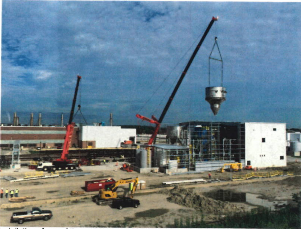
Installation of one of three phosphorus reactors at the Stickney Water Reclamation Plant in Cicero on July 22, 2015. Once in service in early 2016, the phosphorous facility will be the largest of its kind in the world at the largest water reclamation plant in the world.
