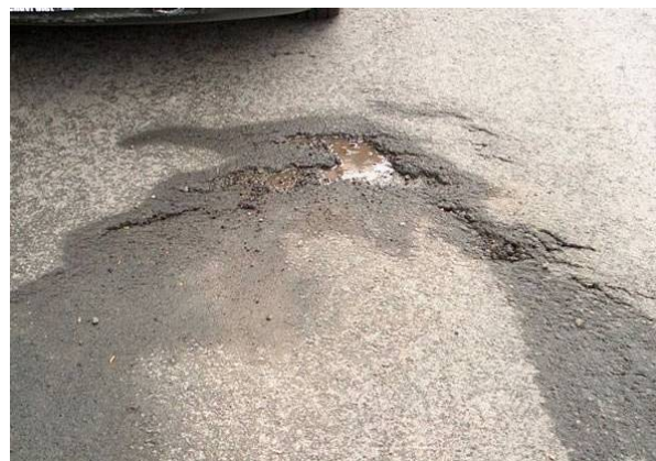
Figure 45. Poor condition of pavement promotes loss of chloride by infiltration to the subsurface. (Photograph by Bob Hodgins)
