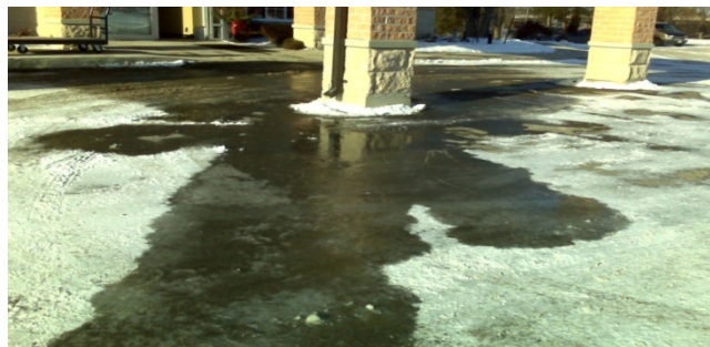
Figure 42. Improperly designed drainage from entrance to nursing home. (Photograph by Bob Hodgins)
