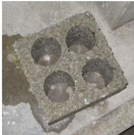
Figure 27. Cores extracted from slabs for material characterization.
