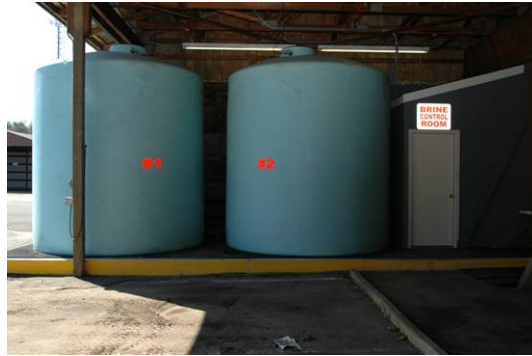
Figure 28. Proper Brine Storage
