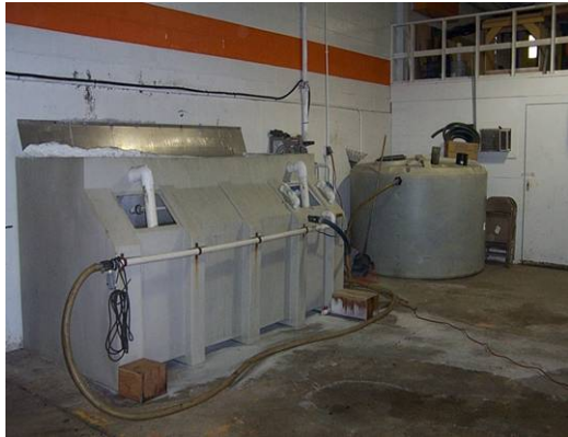
Figure 33. Brine Making Facility
