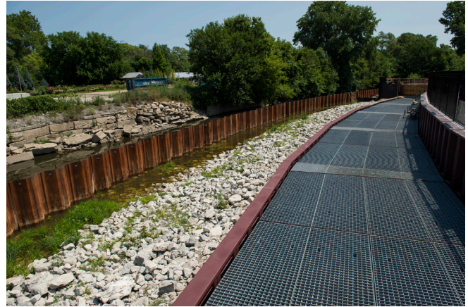
The inlet structure along the banks of the North Branch of the Chicago River will protect the Albany Park community during 100-year rain events by taking on water that climbs above the banks of the North Branch and is then conveyed east 150 feet below Foster Avenue before being released into the North Shore Channel.
