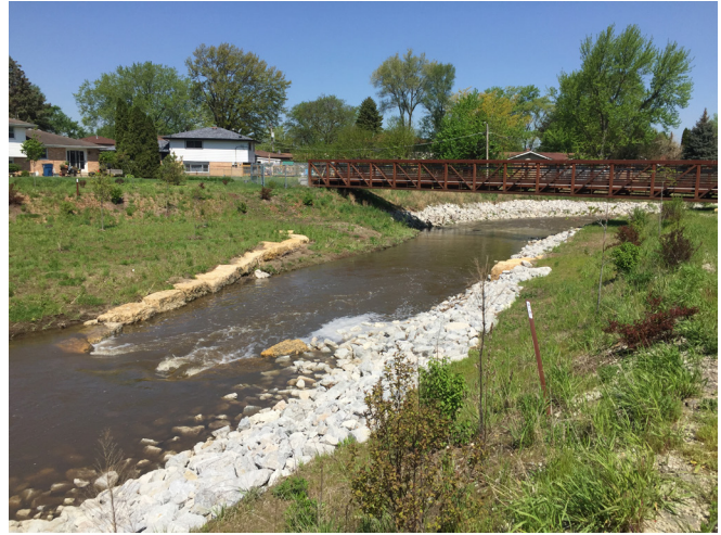
A new pedestrian bridge extends across the restored Tinley Creek in Crestwood. The MWRD restored the waterway with in-stream rock vanes, which provide streambank protection and grade control.
