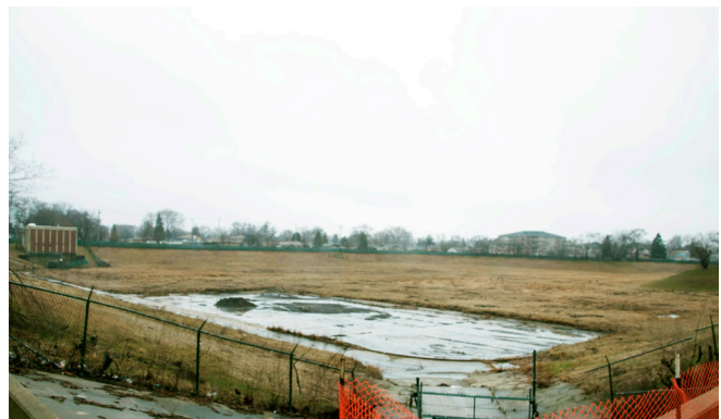
Crews will remove 300,000 cubic yards, or 81,000 tons of dirt in the Melvina Ditch Reservoir by digging down about 11 feet in the current reservoir and another 20 feet down along the new perimeter of the reservoir to build a carefully graded slope that will hold an additional 64 million gallons of water.
