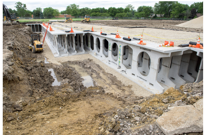
Now covered, the skeletal composition of the new stormwater storage facility under Wescott Park will be the key to keeping the community dry, while conserving water to be reused.
