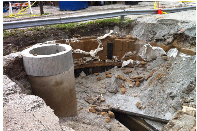
In the photo: The MWRD is investigating damage to a Deep Tunnel structure in Veterans Park in Calumet City.
