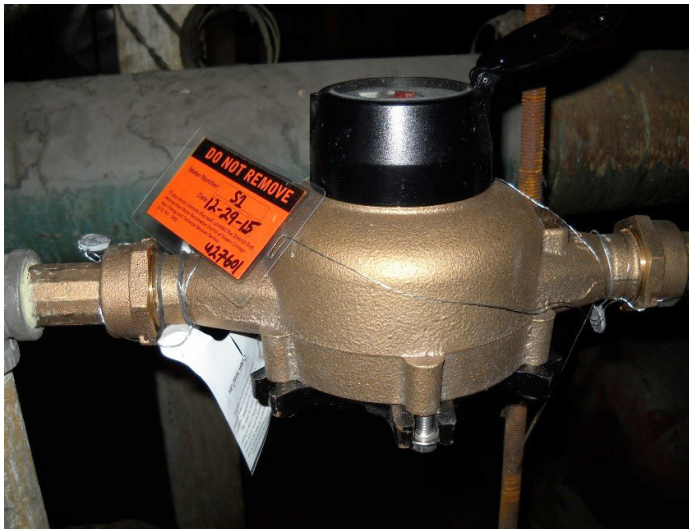
Cold water meter with District seal and label. Photo by Ronald Antequino, Associate Civil Engineer
