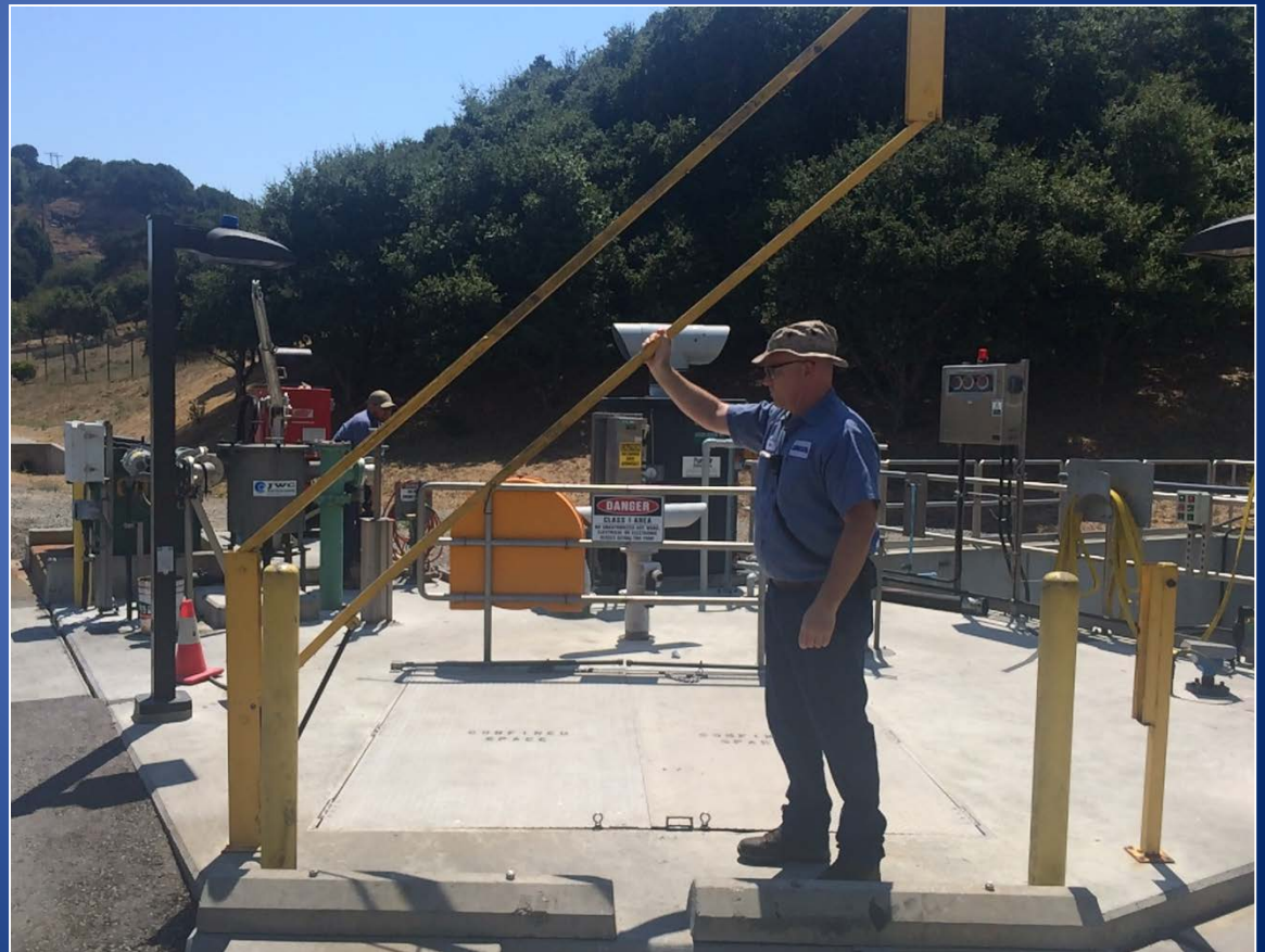
Operator demonstrating Safe Access Gates
