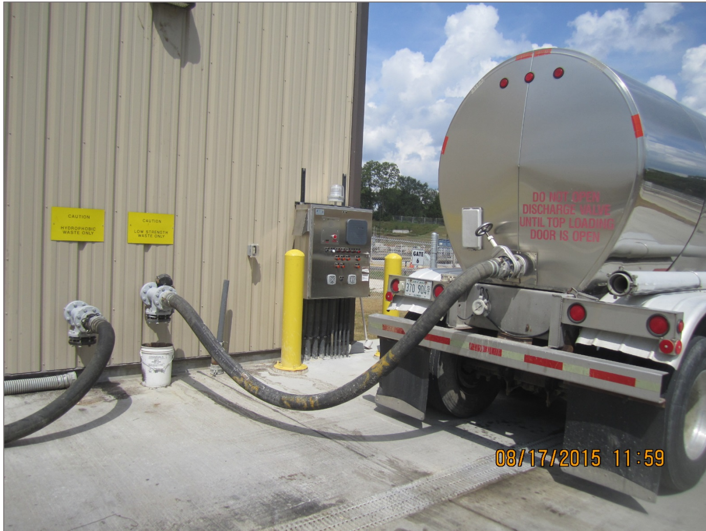
Rock River Water Reclamation District
