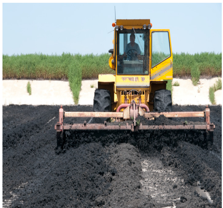
Biosolids processing & drying at Lawndale Avenue Solids Management Area (LASMA).
