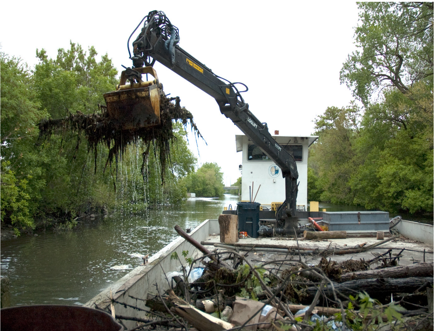
Debris Boat 1 (DB1) with hydraulic crane in action removing debris from the North Branch of the Chicago River.
