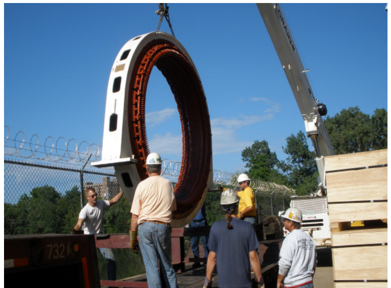
A record breaking weather event caused the world's largest pumping station at Racine Avenue to lose power and ultimately flood in early August. Fourteen 22,000 pound pumps were dismantled, repaired, and reinstalled. Here, MWRD operators carefully transfer a giant stator to a flatbed truck on its way to be refurbished. Diligent and meticulous effort by staff resulted in a restored pump house within 14 days.
