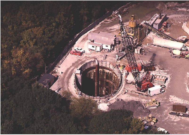
An aerial view shows a construction drop shaft on the District's Deep Tunnel Project. Workers enter the construction area hundreds of feet below ground through this drop shaft and are now finishing the last portion of the project that prevents combined sewer overflows from entering the local waterways. The entire 109.4 mile system will be complete in 2006.
