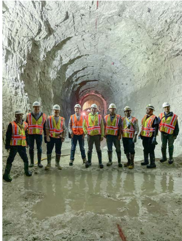
MWRD engineers surveyed excavation progress on the Thorn Creek Connection Tunnel in June. The 22-foot diameter tunnel will convey excess stormwater from Thorn Creek to the MWRD's Thornton Composite Reservoir.
