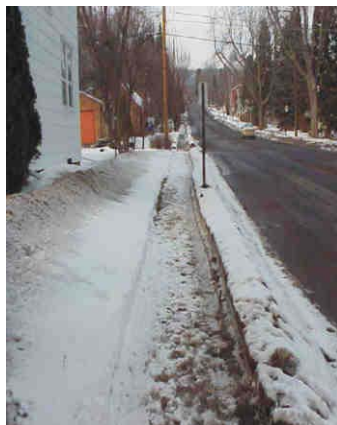
Figure 5-12. Icing behind Curb Drains (City of Duluth, MN).
