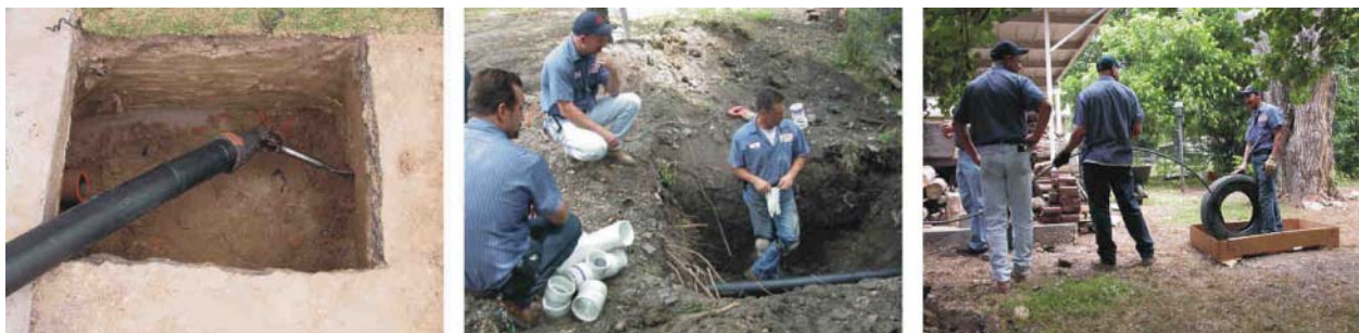
Figure 5-37. Left: Ready for the Pull. Middle: Pipe Moves Quickly. Right: Old Tire As a Container for the Cable (Tric Trenchless Inc).
