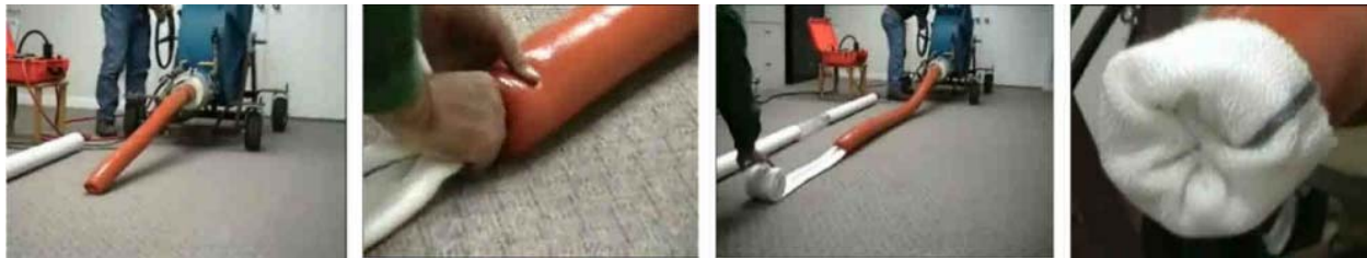
Figure 5-22. Loading of Inversion Drum with Bladder. Left: Extending the Bladder Out from the Drum. Middle Two: Feeding the Liner into the Bladder and Retrieving the Bladder inside the Drum. Right: Liner End Clamped to Invert “Inside-out” (Verline, Inc).
