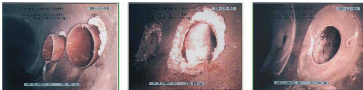
Figure 5-62. Lateral Connection Before, During and After Robotic Repair. Left: Protruding Laterals Before. Middle: The Connections After Grinding. Right: The Connection After the Resin Has Been Applied. (The Janssen Process LLC).
