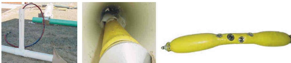
Figure C-24. Push Type Packers. Left: Fitting for Cleanout Installation. Middle: Inside the Lateral. Right: The Packer.
