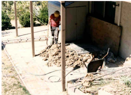
Figure A-124. Difficult Cleanout Location Near the House.
