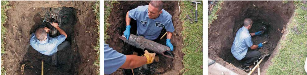
Figure 5-33. Pulling Pit Preparation. Left: Breaking Old Pipe. Middle: Clearing the Way. Right: Remove All Protruding Pipe from the Pulling Wall (Tric Trenchless Inc).
