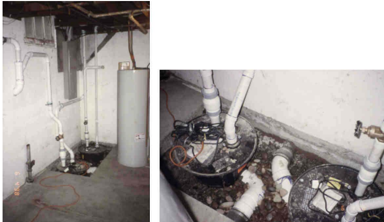
Figure 5-9. Left: Ejector Pumps Installed in the Basement. Right: A Closer View (City of Salem, OR).
