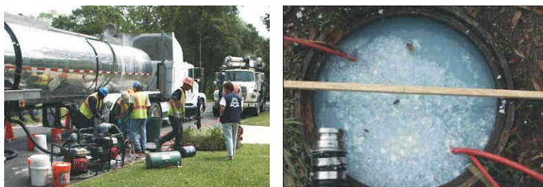
Figure C-25. Sanipor. Left: Truck with Chemicals Near a Manhole. Right: Manhole Filled with a Solution.
