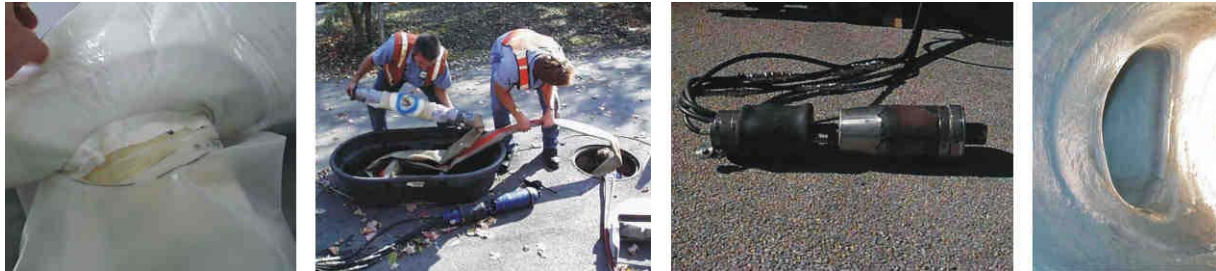
Figure C-15. Left: Liner. Middle Two: Manhole Access; Remote Positioning Device. Right: Installed Liner.
