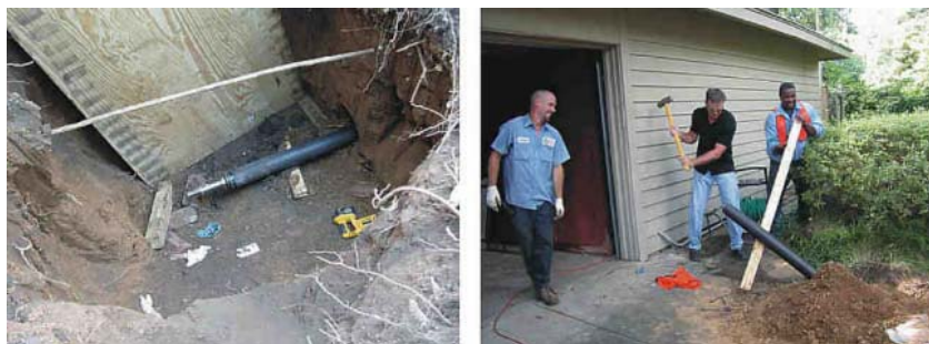
Figure 5-38. Left: Ready to Connect in the Pulling Pit. Middle: “Bumping” in the Entry Pit.
