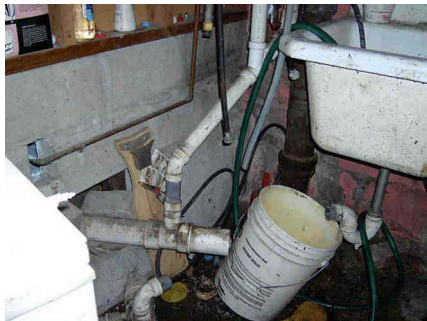
Figure A-32. Cleanout in the House Basement.
