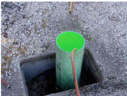
Figure 3-34. Dyed Water in the Stack Monitored for Any Level Drop (City of Key West, FL).
