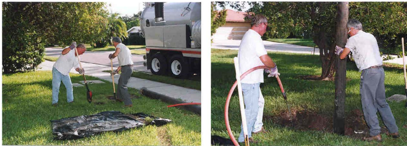
Figure A-78. Installation of Cleanouts at the Property Line. Left: Sod Removal. Right: Pit Hydro Excavating.
