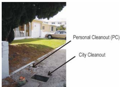
Figure 3-32. Cleanouts on the Lateral Selected for Demonstration of Water Exfiltration Testing (City of Key West, FL).
