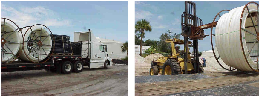
Figure A-83. Replacement Pipe. Left: Delivery to Site. Right: Handling the Pipe.
