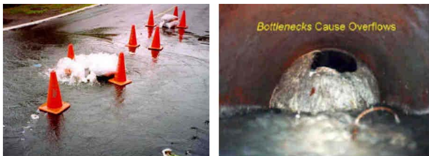
Figure 1-1. Left: SSO at the Manhole. Right: Partial Pipe Blockage (ADS Services).
