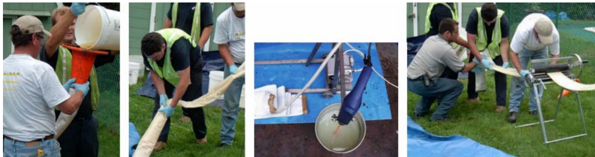
Figure 5-20. Resin Impregnating. Left to Right: Pouring the Resin into the Tube; Manual Resin Spreading Inside the Tube (MaxLiner LCC). Vacuum Impregnation (Easy Liner, Inc.); Calibration Rollers (MaxLiner LCC).
