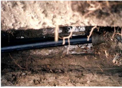
Figure A-129. New HDPE Pipe Extending Beyond Old VCP Pipe—a View from Above.
