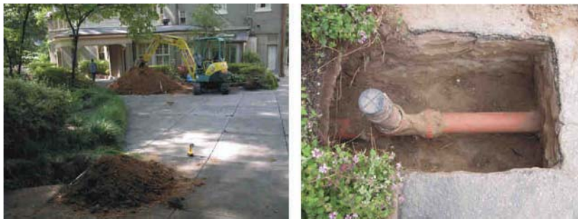
Figure 5-32. Excavating for Lateral Pipe Bursting. Left: Pits Can Be Deep (Roughly 8' Near the House). Right: Shallow Pulling Pit—Approx 2'×4' (Tric Trenchless Inc).
