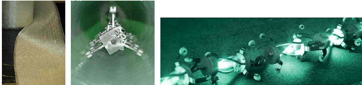
Figure C-4. Left: Tube. Middle: UV-light Source in the Pipe. Right: Several UV-lamps Used for Uniform Curing.
