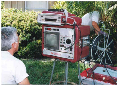
Figure A-79. CCTV Inspection of Laterals from the Pit at the Property Line.
