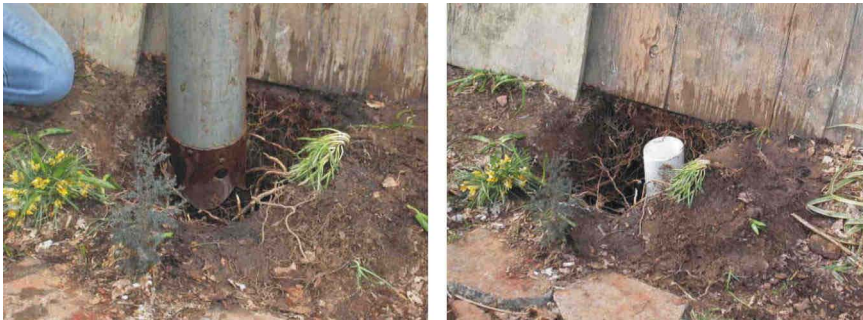
Figure A-17. New Cleanouts. Left: Pit Hydro Excavating. Right: Installed Vac-A-Tee ® Cleanout.
