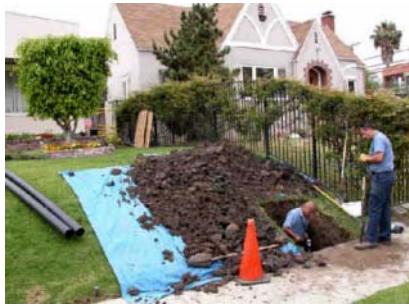
Figure 5-31. Roughly 40' under the Sloping Front Lawn—Suitable for Pipe Bursting (Tric Trenchless Inc).
