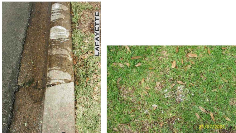
Figure A-100. Left: Exfiltration onto the Pavement (Section #7). Right: Surface Exfiltration onto the Grass (Section #9).
