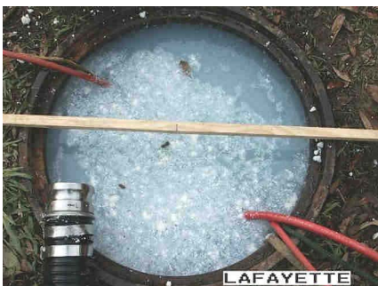
Figure A-99. Manhole Filled with Solution to the Ground Surface.
