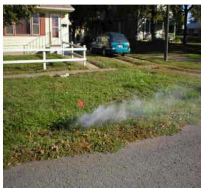
Figure 3-17. Left: Smoke Testing (City of Savannah, MO).
