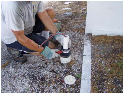
Figure 3-33. Stack over the Cleanout (City of Key West, FL).
