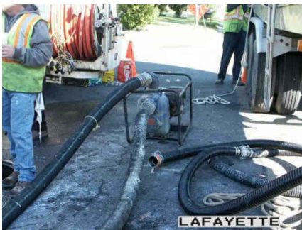
Figure A-98. Pumps.
