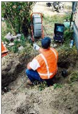
Figure A-1. Inspecting a Lateral with a CCTV Camera Prior to Lining.
