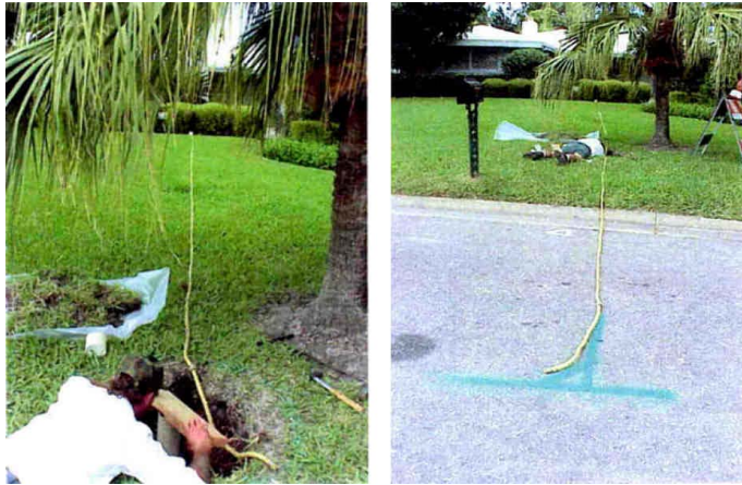
Figure A-81. Improved Recording Technique During Locating of Laterals. Left: Lateral Marking Rope Laid on the Ground. Right: Rope Extending from the Mainline.
