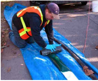
Figure A-53. Using a Roller to Spread the Resin along the Liner.
