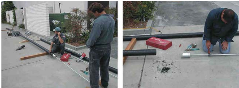
Figure 5-35. Bead Reaming. Left: Bead Reamer Aligned with the Pipe. Right: Shaved Bead Removed by Reamer Blade (Tric Trenchless Inc).
