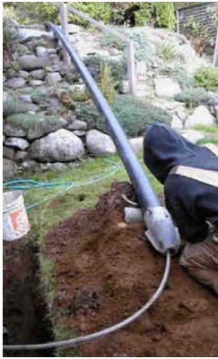
Figure A-72. Bursting Head Attached to the Replacement Pipe and the Pulling Cable Near the Entry Pit.
