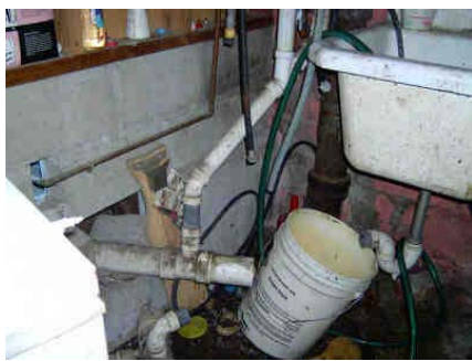
Figure 5-17. Cleanout in the Basement (City of Weymouth, MA).
