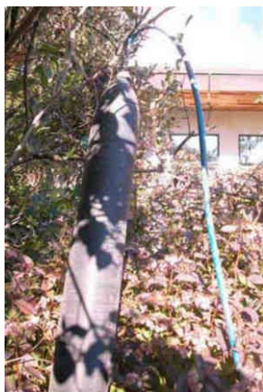
Figure A-58. Excess Bladder Extending out of the Trench with Air-pressure Hose Connected.
