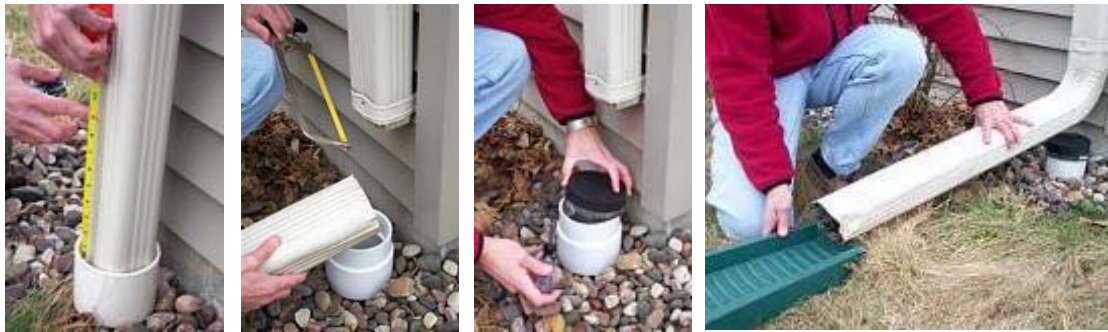
Figure 5-1. Downspout Disconnection (Milwaukee Metropolitan Sewerage District, WI).
