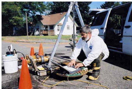
Figure A-15. Flow Monitoring.
