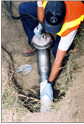
Figure A-9. Calibration Tube Being Checked for Holding the Pressure.
