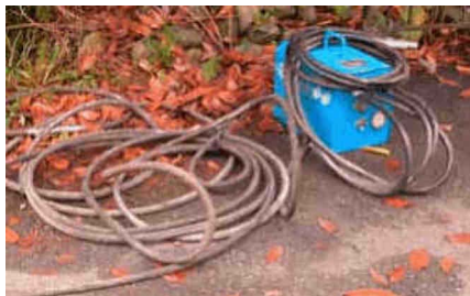
Figure A-63. Control Box and Hydraulic Lines.
