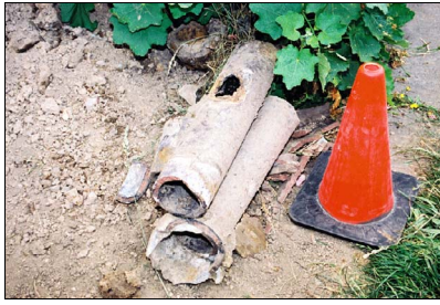
Figure A-2. Example of the Condition of Laterals that Were Relined.
