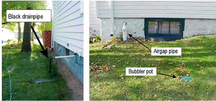
Figure 5-10. Surface Discharge of Disconnected Flow. Left: Black Drainpipe. Right: Bubbler Pot (City of Duluth, MN).
