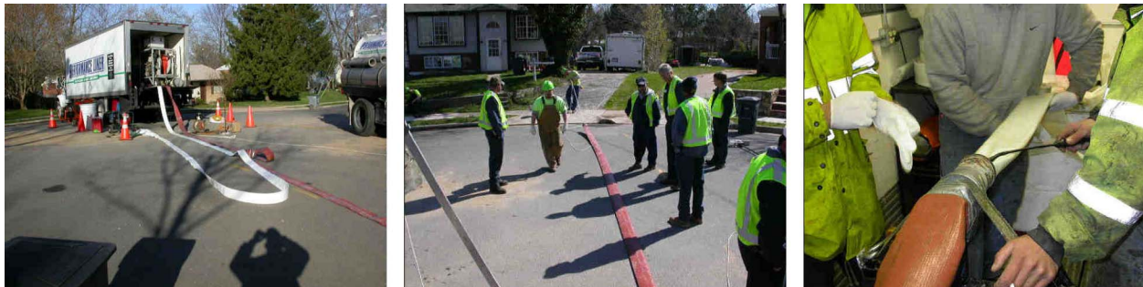
Figure A-23. Pulling the Liner/Bladder Assembly into the Launcher. Left: Both Tubes Laid Out on the Ground. Middle: Pulling the Cable Inside the Launcher. Right: The Assembly Entering the Launcher.
