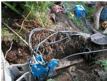
Figure A-71. Hydraulic Lines Attached to the Control Box.
