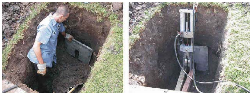
Figure 5-36. Pulling Pit. Left: Placing the Bearing Plate. Right: Pulley and Ram (Tric Trenchless Inc).
