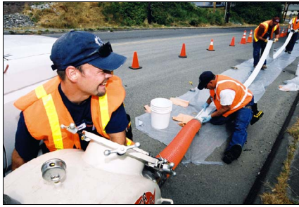
Figure A-6. The Crew Reeling the Resin-saturated Liner into the Air-inversion Machine.
