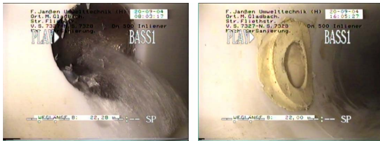
Figure 5-61. Robotic Repair Stops Infiltration. Left: Infiltration Before Repair. Right: Repaired Connection. (The Janssen Process LLC).
