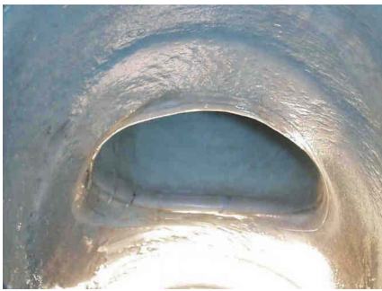
Figure A-28. Installed T-liner at the Lateral-to-mainline Connection (a View from the Mainline).
