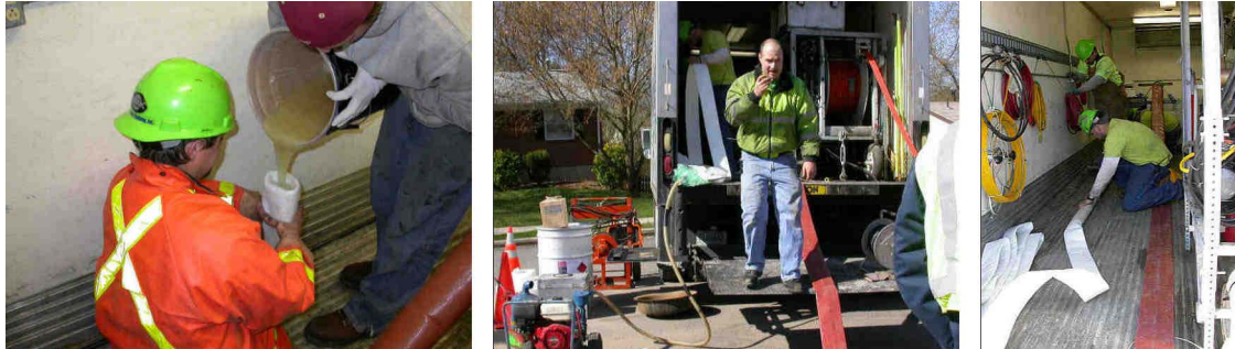
Figure A-22. Liner Impregnation with Resin. Left: Pouring the Resin into the Tube. Middle: Vacuum Hose Connected to the Tube. Right: Vacuum Impregnation.
