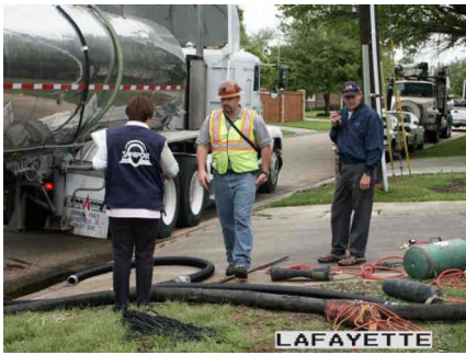
Figure A-97. Hoses for Pumping the Chemicals.
