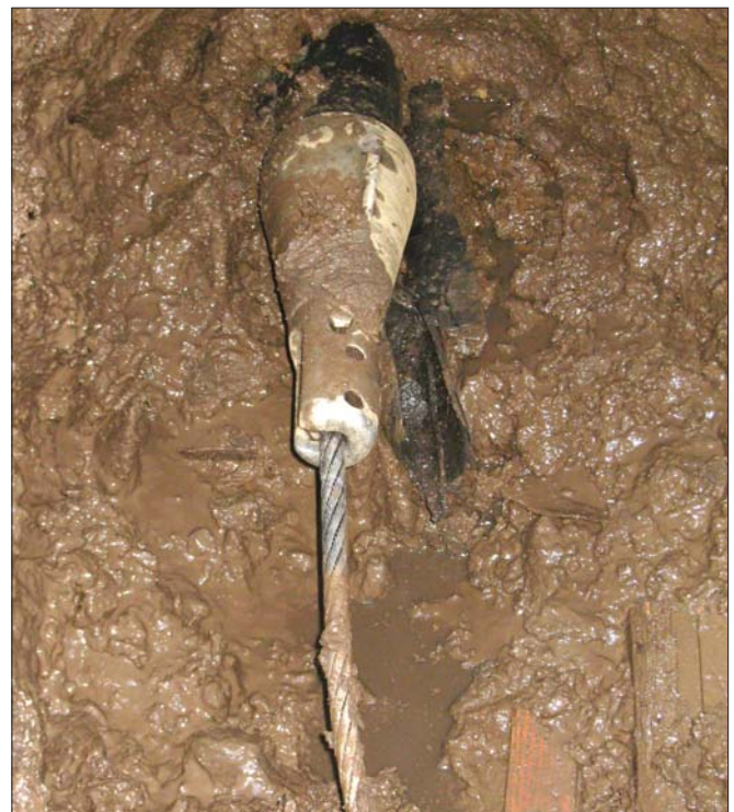
Lateral bursting is a much less intrusive replacement process compared to open-cut replacement.
