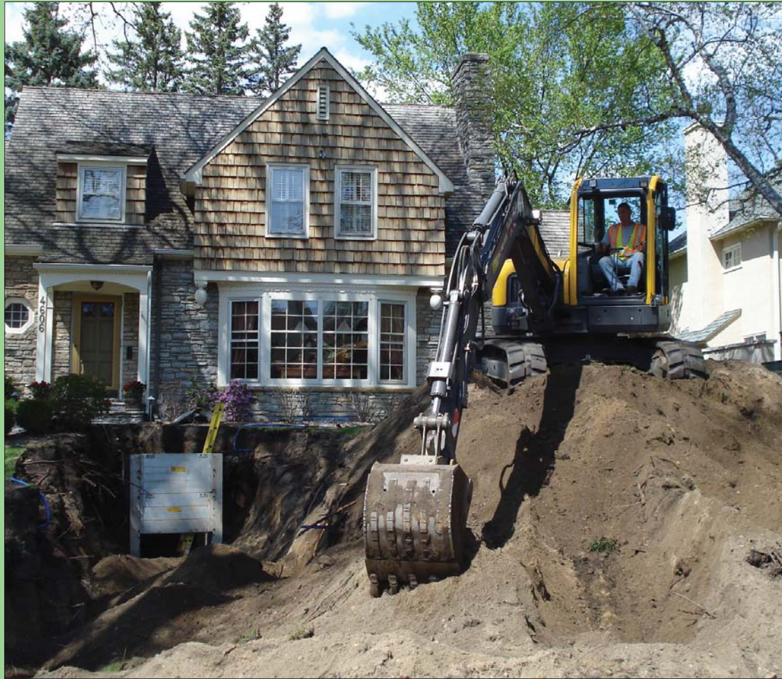
Lateral replacement can be a nightmare for homeowners when trenchless methods aren't utilized to minimize disruption.
