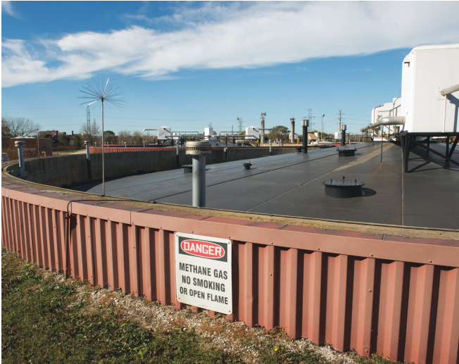
Anaerobic digesters produce biogas for energy production at the Calumet facility.
