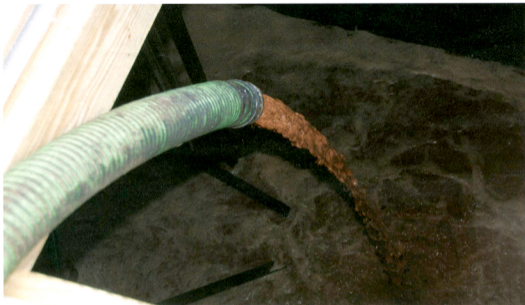
Brewery waste, a high-strength organic material, is transferred into an MWRD distribution chamber. This waste will improve and stabilize the MWRD's enhanced biological phosphorus removal process during treatment.
