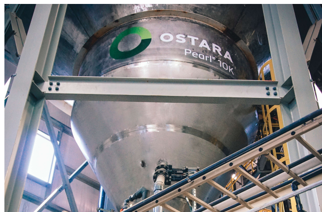
One of the three reactors installed at the world's largest phosphorus recovery facility at the Stickney WRP.
