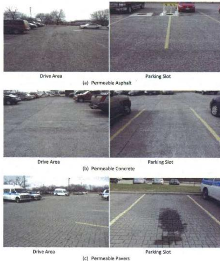
Picture 3. Pictures of permeable parking sections (a) asphalt, (b) concrete, and (c) pavers taken in December, 2012 showing deterioration of surface in driving areas as compared to parking slots.
