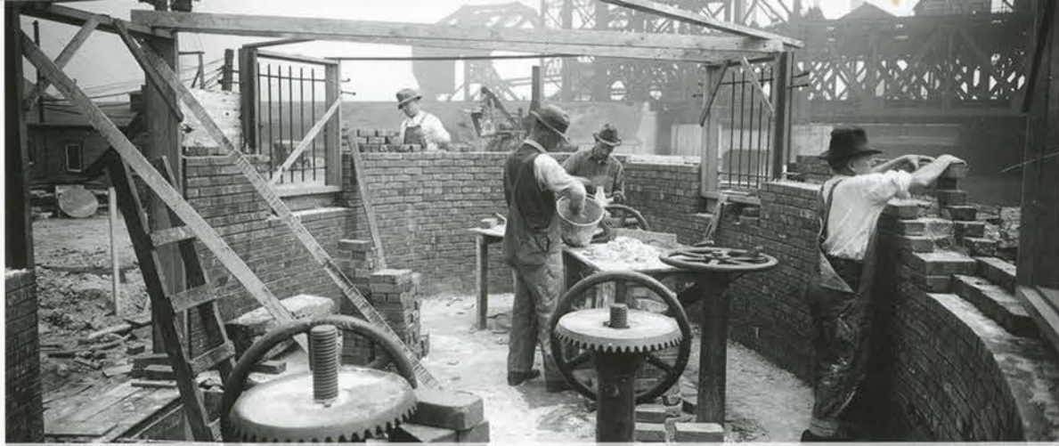
Masons build a headhouse for the Calumet intercepting sewer system on June 13, 1923.
