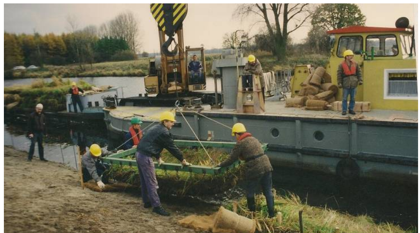
Placement of individual vegetated revetment modules is easily accomplished when using a crane and requires little manual labor.
