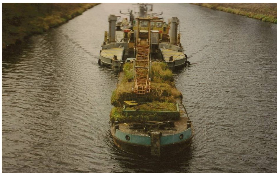
When installed on riverbanks and canals, transport and installation is often times best accomplished through the use of a barged equipped with a crane.
