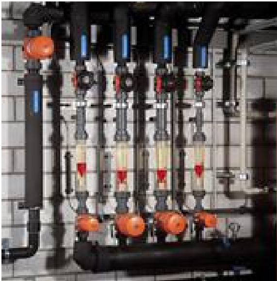
Sodium Hypochlorite Disinfection
