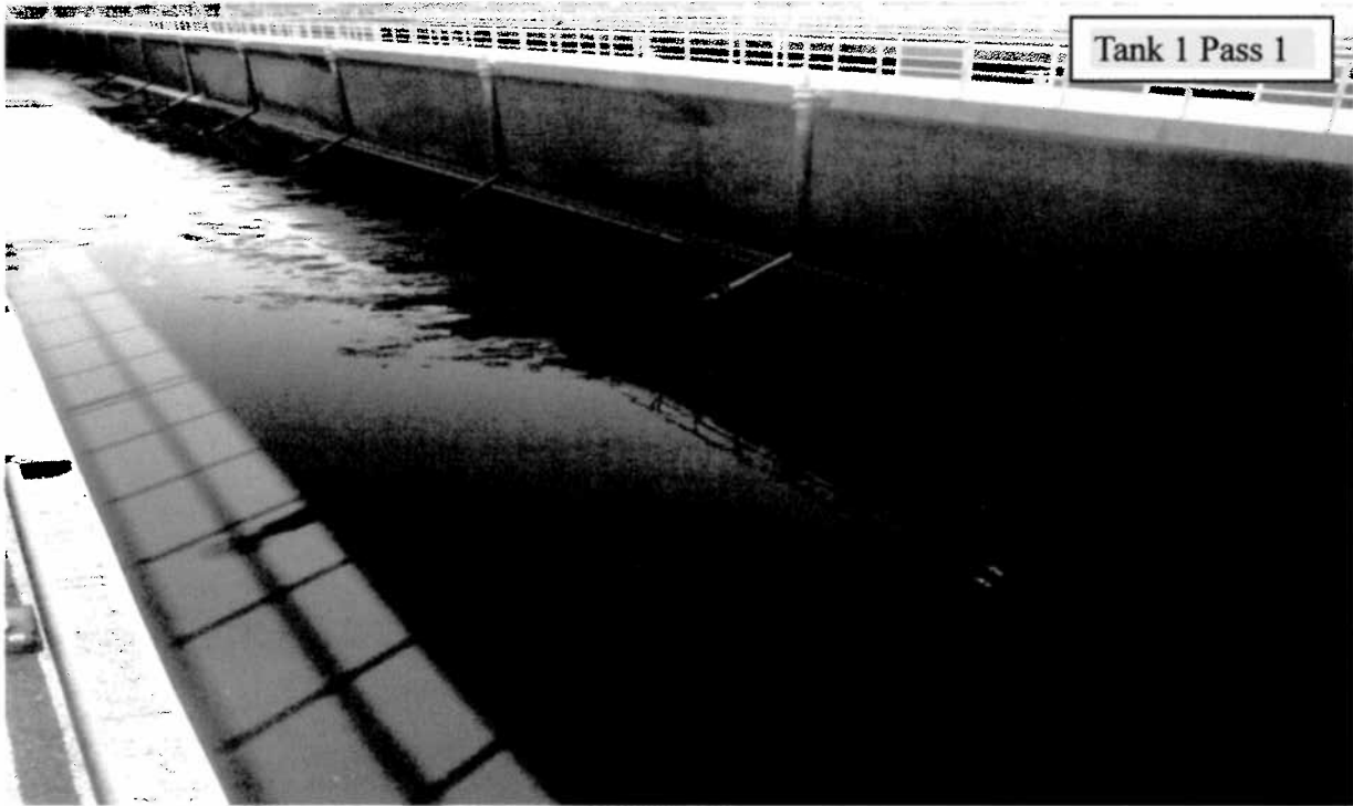
FIGURE 3: PHOTOS OF AERATION TANKS 1 AND 4 - PASS 1 AFTER DEPOSITION STUDY WITH CAPTURE DRAINAGE
