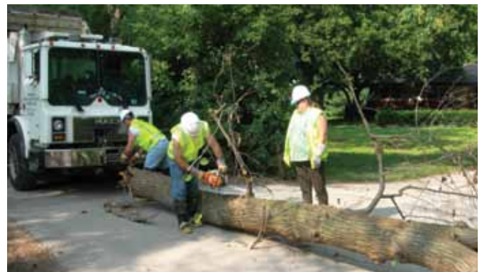
District personnel remove trees, cut them up into manageable pieces and transport them to a disposal site.
