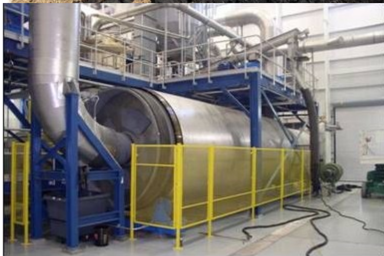
Rotary drum dryer, South Cary, NC
