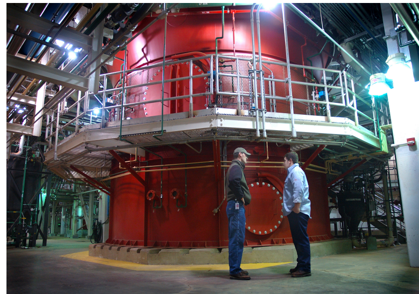
Wastewater solids (SSI) incinerator, St. Paul, MN
