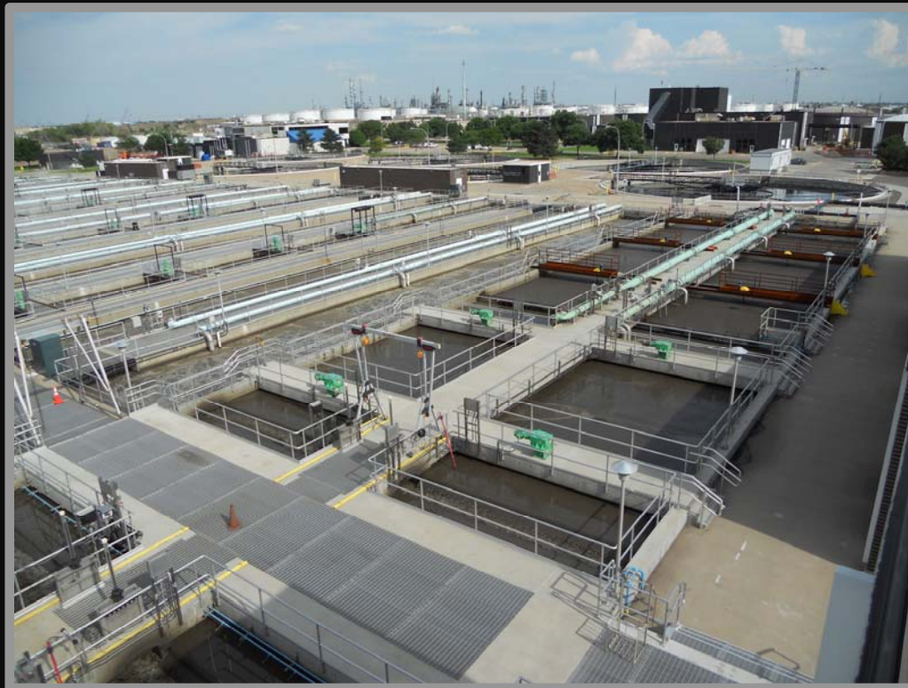
Two Anaerobic RAS Reactors
