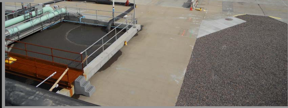
Temporary Gravity Thickener Overflow Feed
