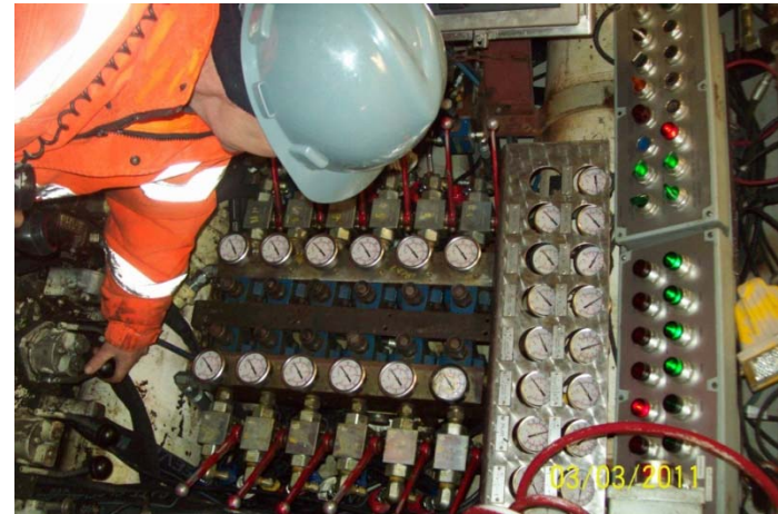
Hydraulic Pressure Controls
