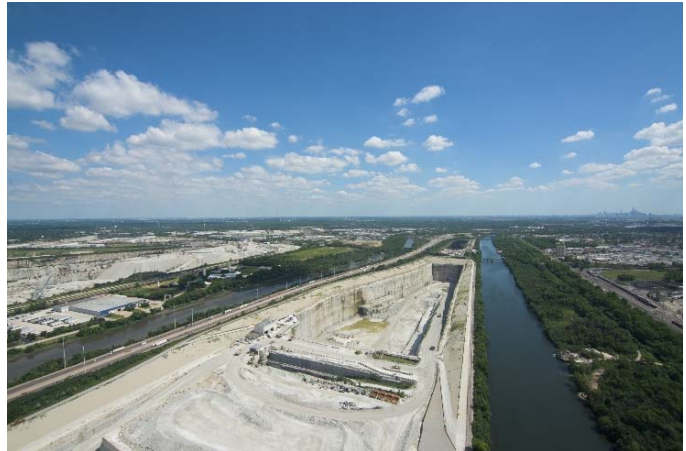
The first stage of the McCook Reservoir opened on December 4, 2017, providing 3.5 billion gallons of storage capacity. The final stage of the TARP system is scheduled to be completed in 2029.
