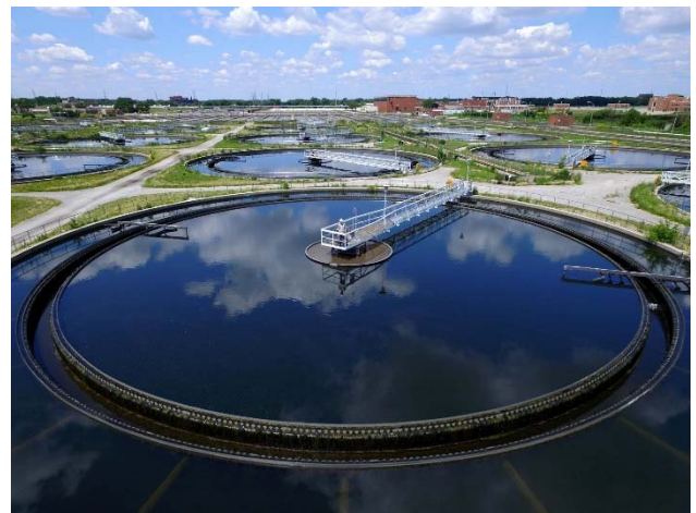
Settling tanks at the Calumet Water Reclamation Plant.
