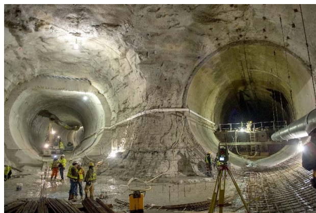
Construction at the confluence of the McCook Reservoir Connecting Tunnel (left) and Mainstream Tunnel (right).
