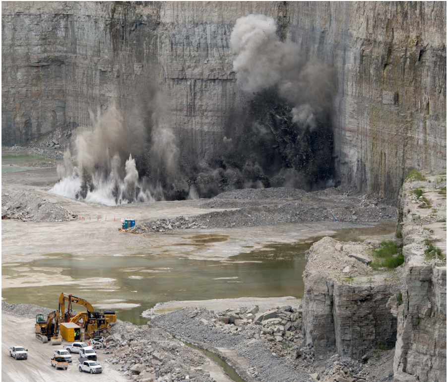
Excavation of a 230' x 130' area at the McCook Reservoir began with a bang as 28,000 lbs. of explosives, requiring 996 detonators, were used to remove over 27,000 tons of limestone.
