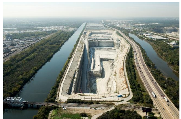
Facing Southwest in Bedford Park, the future McCook Reservoir will service 3.1 million people in 37 communities providing a total volume of ten billion gallons. The reservoir is planned to be completed in two stages. The first stage (shown in the foreground) will provide 3.5 billion gallons of storage and is expected to be completed in 2017. The second stage (shown in the background) will provide 6.5 billion gallons of storage and is expected to be completed in 2029. The McCook Reservoir is projected to bring $90 million/year in flood reduction benefits to its residents.
