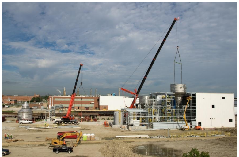
Construction of the phosphorus recovery facility at the Stickney Water Reclamation Plant.
