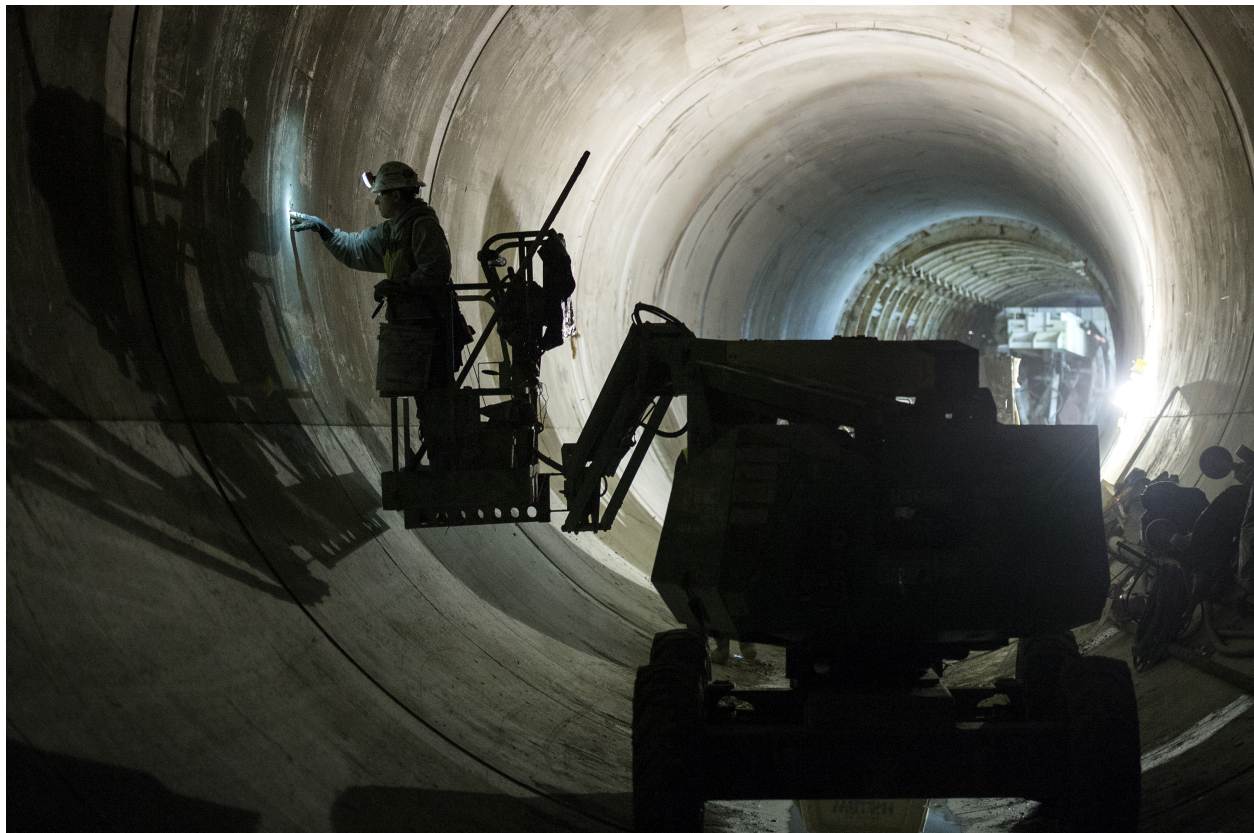
Work continues on construction of the Des Plaines Connecting Tunnel near the MWRD’s Mainstream Pumping Station and McCook Reservoir in March.
