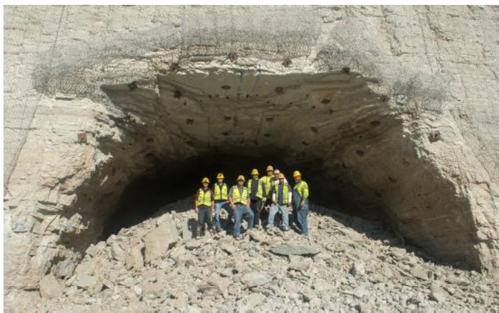
Workers gather for a unique portrait opportunity near the entrance to one of the tunnels at the McCook Reservoir, standing on some of the 4,600 tons of rock that had been blasted out using 1,000 tons of explosives. The blast opened the top portion of the 33-foot diameter tunnel to the reservoir. Work remains to be done before the first stage of the 10 billion gallon reservoir becomes operational in 2017, but the McCook Main Tunnel is now open to the reservoir. A major part of the Tunnel and Reservoir Plan (TARP), the McCook Reservoir will help reduce flooding and improve water quality within a 254.7 square mile area, including much of the city of Chicago and 36 other communities.
