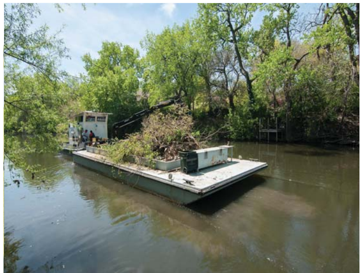
The MWRD handles large debris removal and sidestream cleanup projects along the North Shore Channel, the Cal-Sag Channel and the Chicago Sanitary and Ship Canal using debris boats and pontoon boats. Debris Boat 1 (DB1) is pictured at work on the North Shore Channel.
