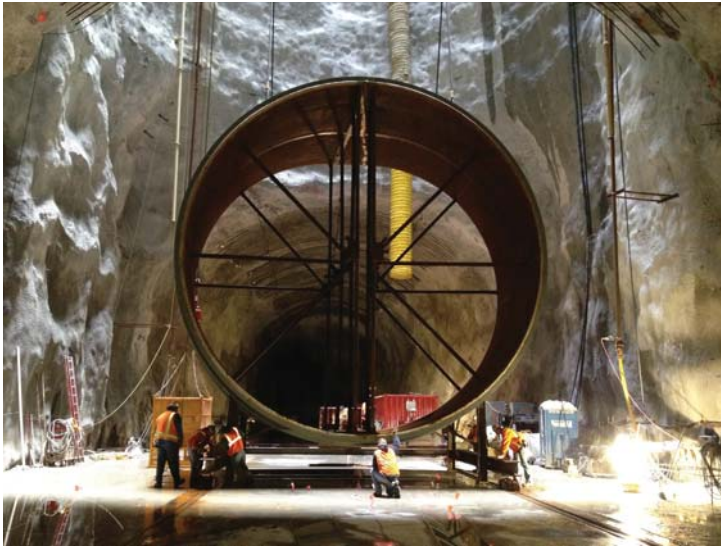
The first of several sections of steel liner is lowered more than 300 feet below ground into a portion of the tunnel connecting the Calumet TARP tunnel system and the Thornton Composite Reservoir. The 30 foot diameter liner weighs 220,000 pounds.
