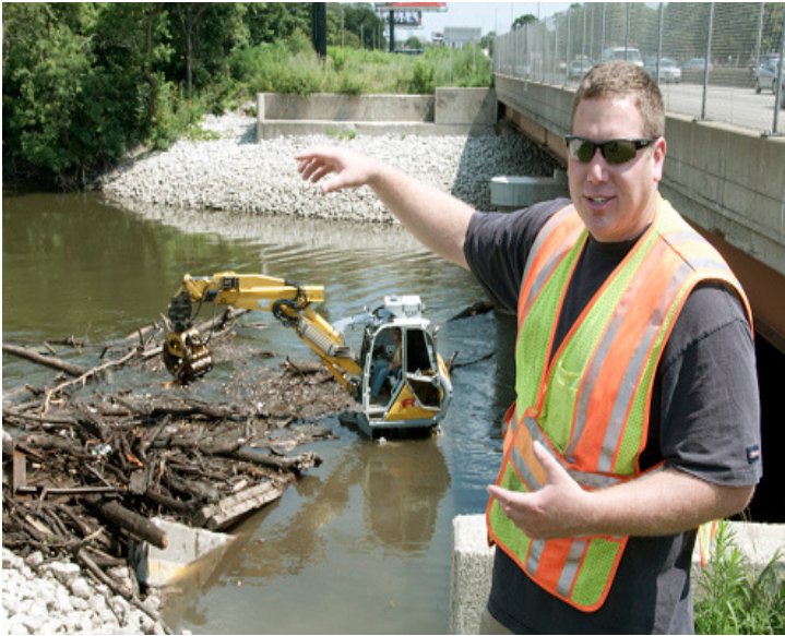
MWRD Senior Civil Engineer and Small Streams Management Program Manager Brian Levy, at a project site in Maywood, discusses the methods employed by his crews to secure and remove debris from a large waterway.
