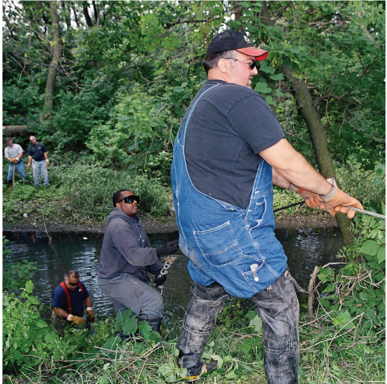
District Personnel perform channel maintenance to remove large tree branches and other debris from inland waterways, providing relief to areas affected by overbank flooding.
