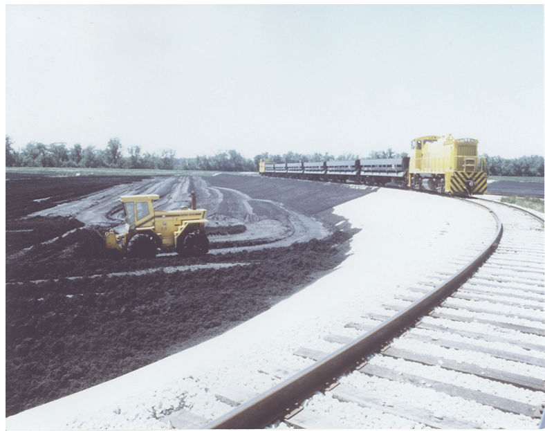
Biosolids are transported from the Central (Stickney) Water Reclamation Plant to nearby drying beds. Once the drying is complete, the biosolids are recycled into landfill.
