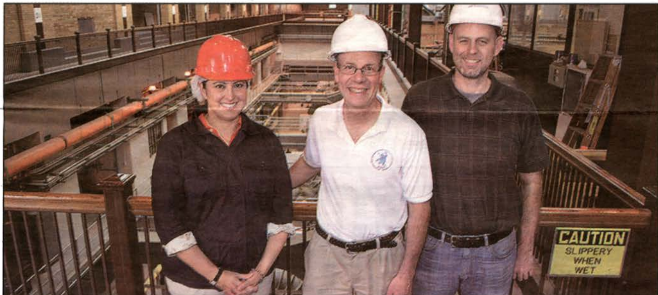
MWRD Board of Commissioners President Mariyana T. Spyropoulos stands in front of six mammoth pumps—originally built and installed in 1939—with Brett Garelli (center) and Joe Cummings. Group tours are available at the plant. For more information, visit mwrdd.org and click on the "Tour Information" icon. — Archer Journal News photo by Tim Hadac
